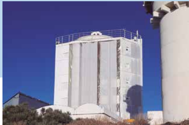
Figure 2: GREGOR panel refurbishing: new facade (left part), work in progress (middle part) and previous panels (right part).
